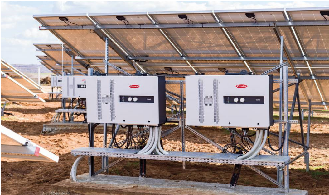
Figure 7: AC daisy-chaining with Fronius Tauro ECO in a decentralised group configuration
