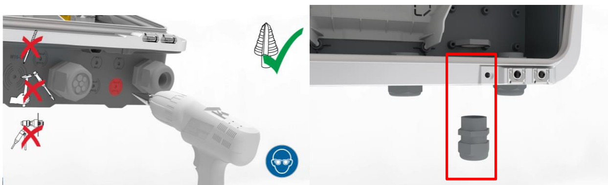
Figure 3: Drilling through the base shell and PG screw fitting inserted at the drilled-through point
